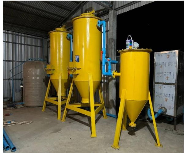
Fig.2: Side view of the desulfurizing system at Heng Mean farm in Kampong Thom province
