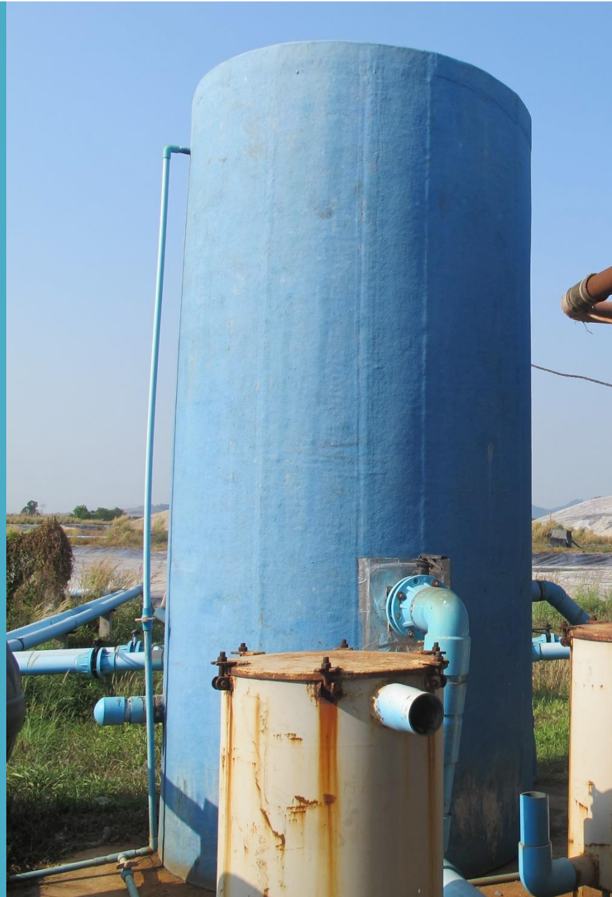
Fig. 1 Old and ineffective desulfurization system at M's Pig Farm
