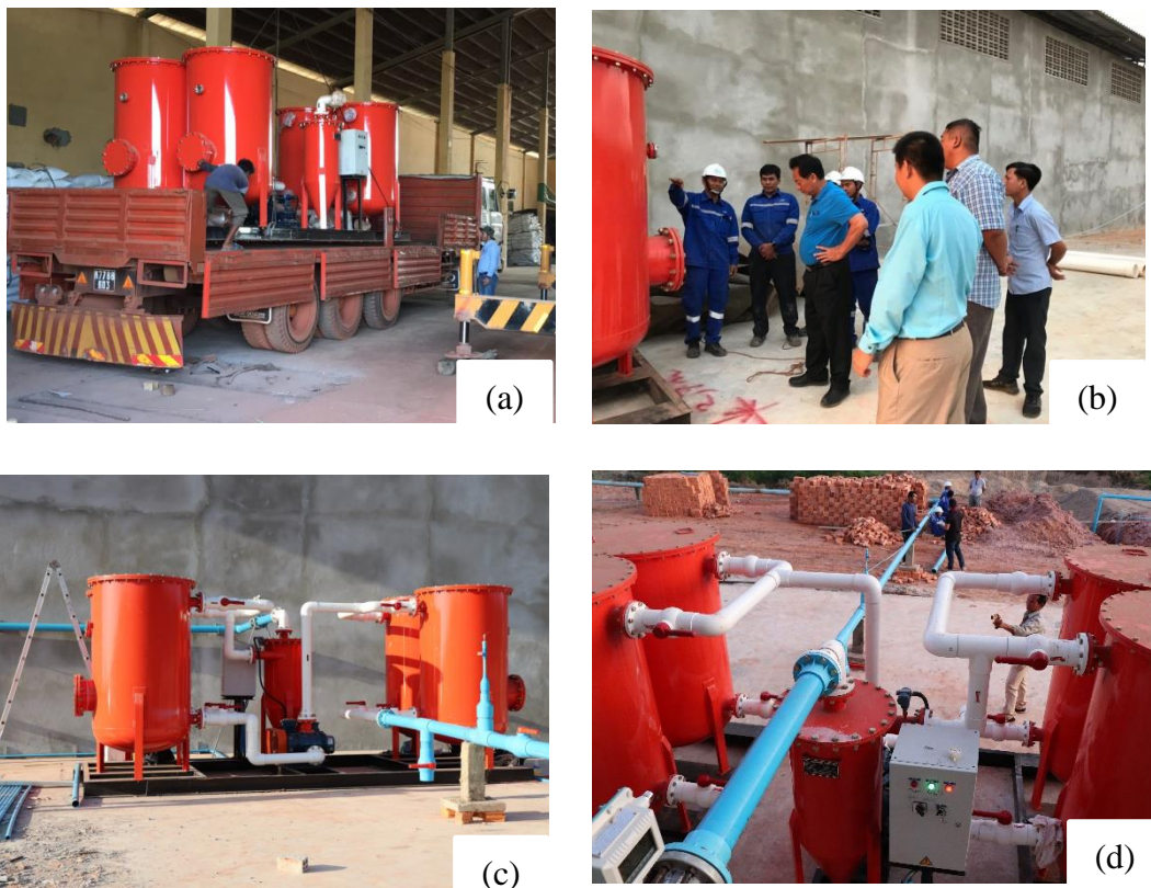
Fig. 2 Installation of desulfurization system at M's Pig Farm (a) arrival of the equipment, (b) installation activities, (c) finished installation, and (d) commissioning/operating
